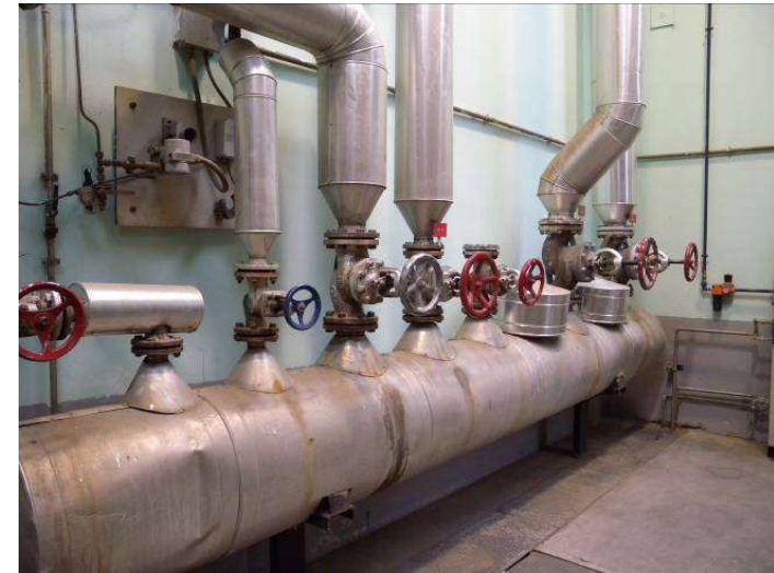
Insulated steam pipe
